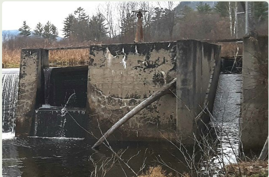
East side of dam looking upstream at stopboards (left) and fish ladder (right)
